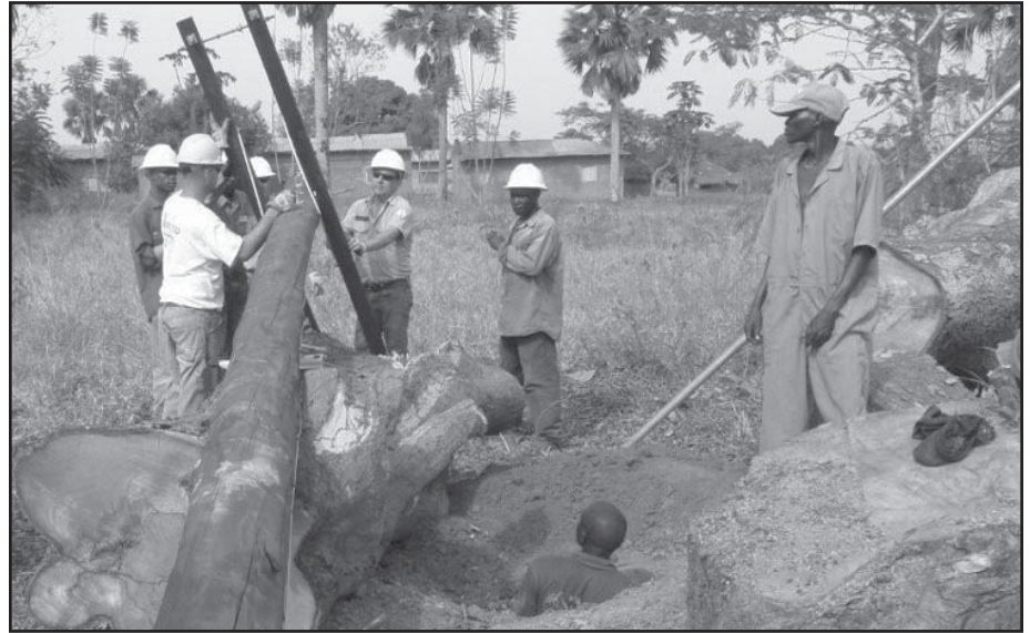
All line work in Sudan is done by hand — even digging pole holes.
