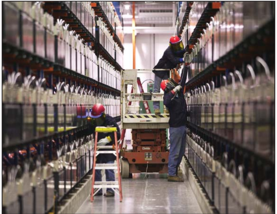
Golden Valley Electric Association, based in Fairbanks, Alaska, uses the world's most powerful nickel-cadmium battery to hedge against power outages. When needed, the 13,760-battery cell system can provide 27 megawatts of power for 15 minutes. — Courtesy of Patrick J. Endres/Alaskaphotographics.com
