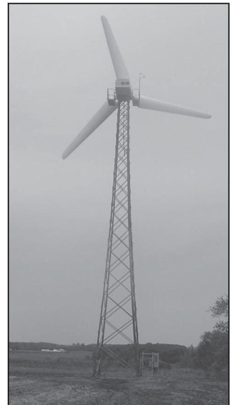
This Jacobs 31-20 kW wind turbine received a $17,500 USDA grant.
