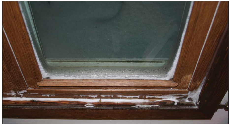
Frost buildups like this can be a sign that your windows could benefit from being sealed with caulk. Look for these air leaks now.
