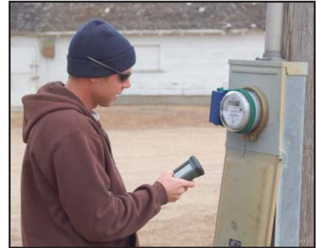
Federated reached a milestone December 22. The last main meter was changed out to the new electronic automated meter reading (AMR) system. The last meter was installed in the town of Wilder. Federated Journeyman Lineman Matt Madden programs one of the final installs. ♻️
